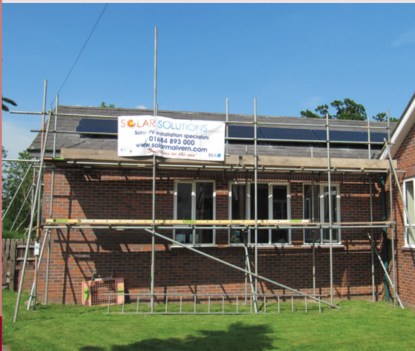
Colwall Village Hall with solar panels installed
